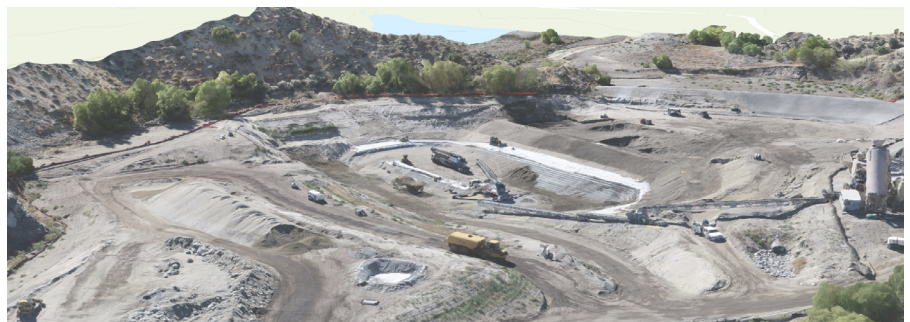
Drone 3D image showing construction at the Littlerock Dam grade-control structure in 2019.
