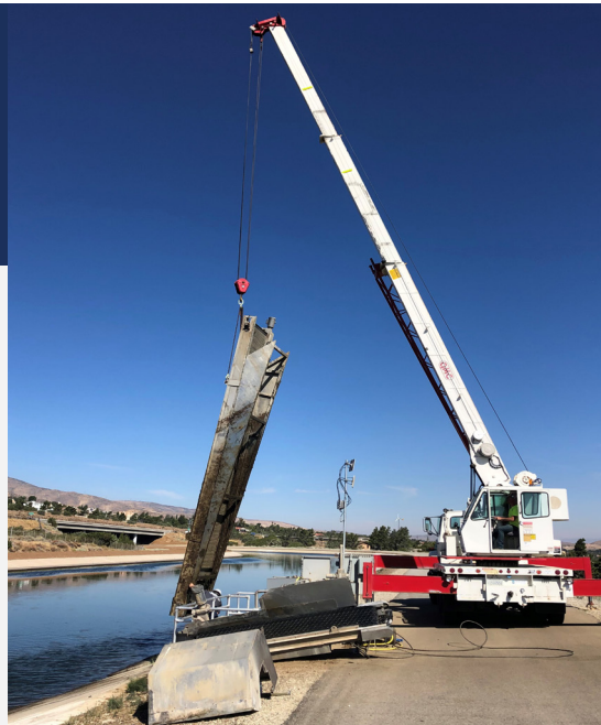
The traveling screen is lifted out of the aqueduct for repairs and cleaning.
